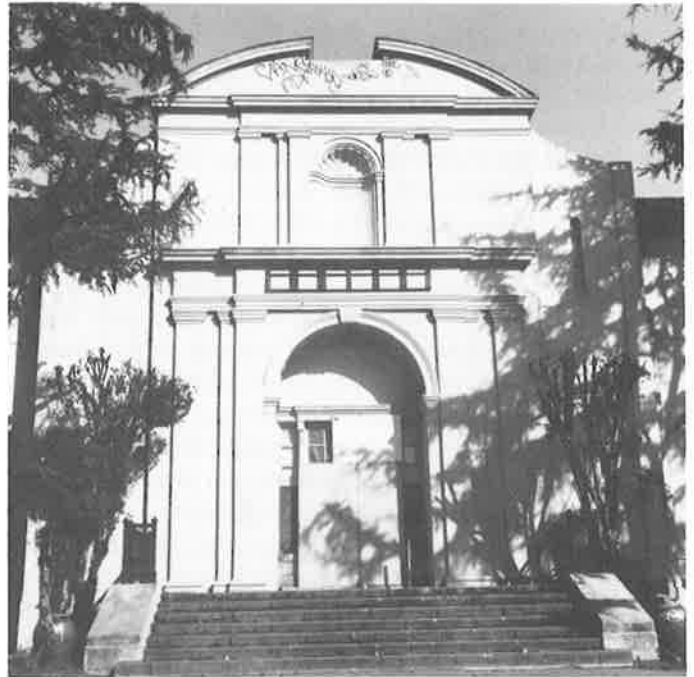
University High School-Merritt College building shows evidence that site security is less than perfect. Negotiations with Children's Hospital may offer hope. (Phil Bellman)
