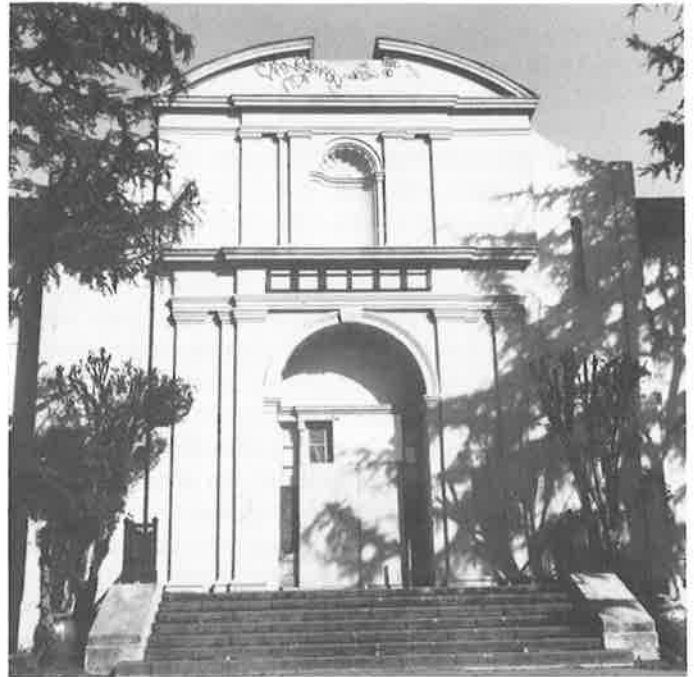
University High School-Merritt College building shows evidence that site security is less than perfect. Negotiations with Children's Hospital may offer hope. (Phil Bellman)
