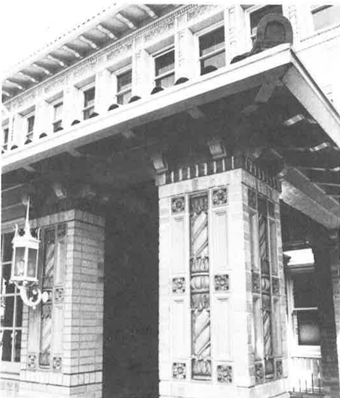
Rich detailing in brick, terra cotta, wood, and metal, at King's Daughters Home on Broadway, 1912ff. (Phil Bellman)
