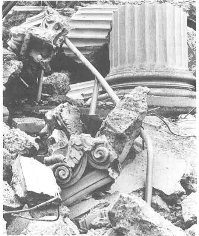
Fourth Church of Christ, Scientist: Two-year controversy enlisted National Trust support, prompted preservation task force, put OHA on the map at City Hall. (Phil Bellman)
