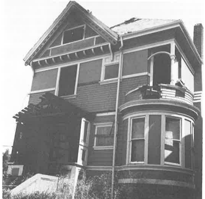
Simpson House, 524 23rd St., illustrates typical sequence of events--vacated, then stripped of ornament, then burned;
