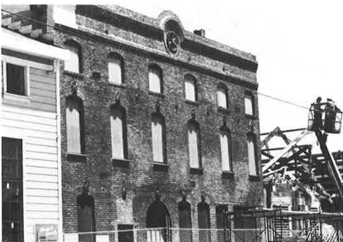
Oakland Ironworks: demolition of brick buildings in progress (frame building to left has been landmarked and rehabbed) (Leslie Flint)
