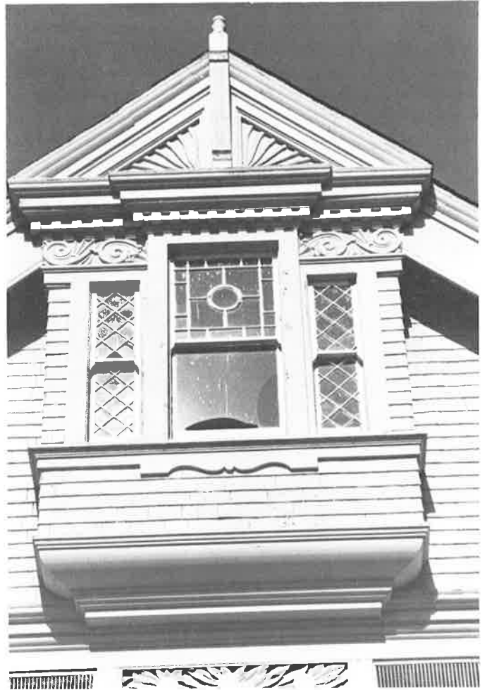
Herrick House, Hawthorne & Webster. The OEDE plans to move this 1885 house, designed by well-known architect Clinton Day, to Preservation Park (Phil Bellman)
