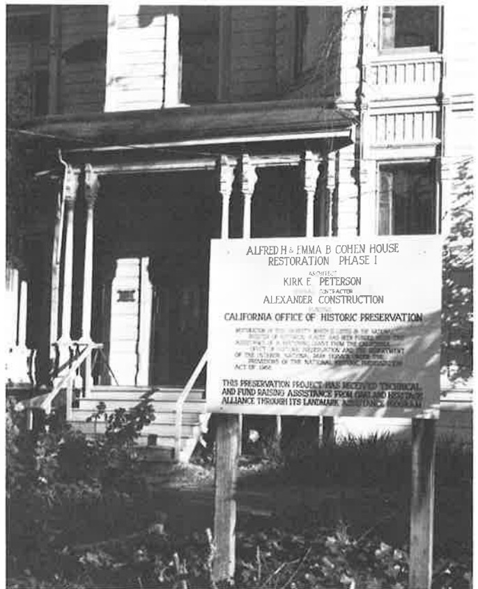
Phase I of the Cohen House restoration is underway thanks to numerous local contributors who made the federal matching grant possible.
