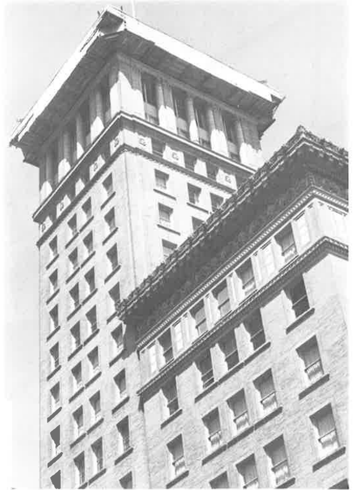
Deteriorating architectural terra cotta on the Bank of America Tower at 1212 Broadway may be replaced later this year.
