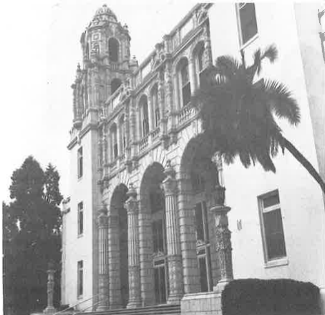
The magnificent facade of the original Highland Hospital administration building is threatened by plans to expand parking facilities.
