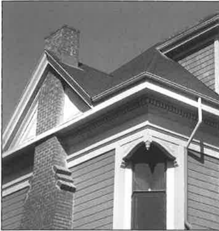
ROOF DETAIL of a building in Preservation Park, the focus of the July 23 tour.
