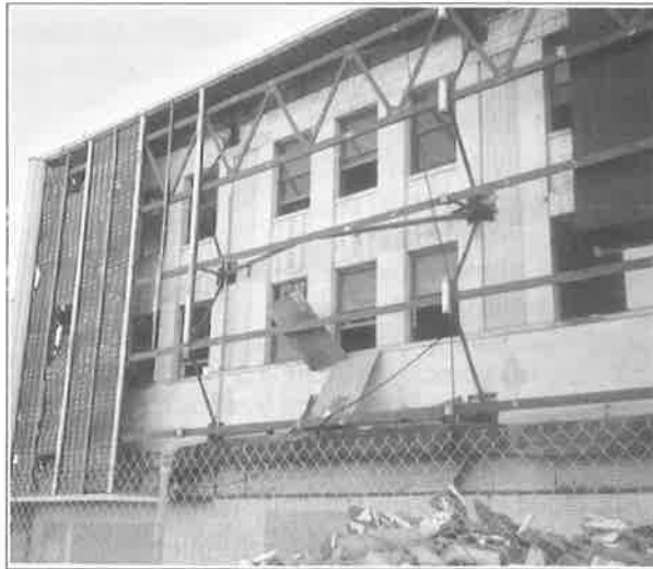
The 1964 metal facade is removed from the Sears buildings, revealing the intact original Art Deco exterior. (Joyce Roy)
