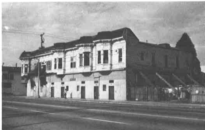
Hinson Building at 11th Ave. and East 12th St. In addition to the fire damage, the building has serious structural problems as indicated by the diagonal buttresses along the side lot line.
