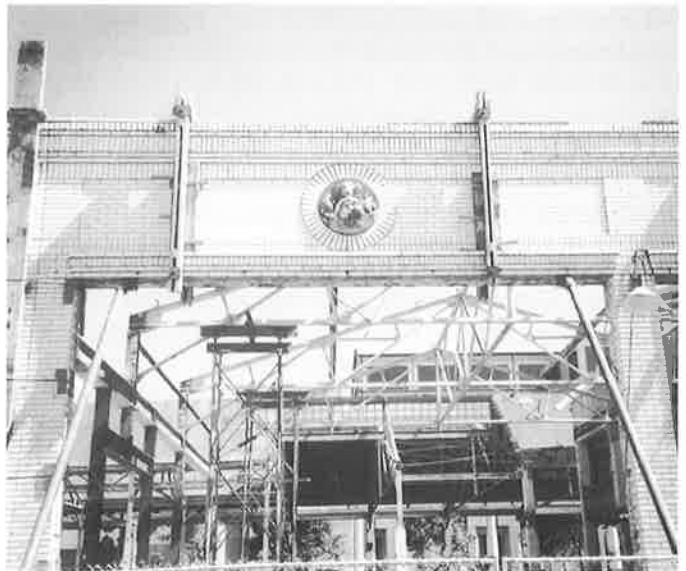
Swan's Market, taken down to its bare essentials. When rebuilt, it will be a single structure with homes, businesses, and open space. EBALDC plans fundraising for historic and aesthetic extras. (Carolyn Douthat)
