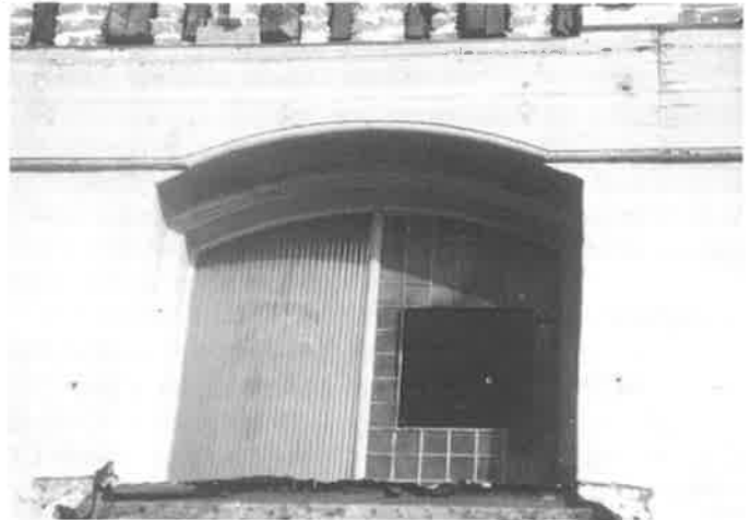
Original ground floor window arches surfaced during work on the much-remodeled Dahlke's saloon in Old Oakland, illustrating once again the value of exploratory demolition. (Betty Marvin)
