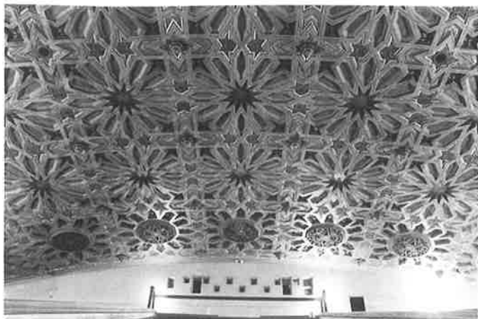
Board is concerned that ornate gilded plaster ceilings in the Fox Oakland Theater - one of the Magnificent Seven - are vulnerable to damage if roof is not maintained. (Fred Reichman)
