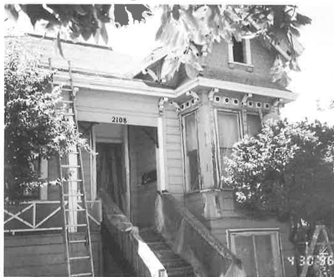
Plastic sheeting on doors and windows will help keep lead dust out of this Victorian cottage while exterior work is done. In 1905 Oakland architect A.W. Smith cited as an advantage of shingled Craftsman houses that they did not need "a thin film of lead poison" every two years. (ACLPPP)
