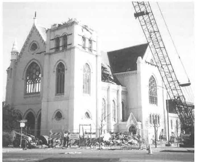
Demolition of St. Francis de Sales Cathedral in 1993 was a major change on San Pablo Avenue. For more, visit the exhibit. (Don Hausler)
