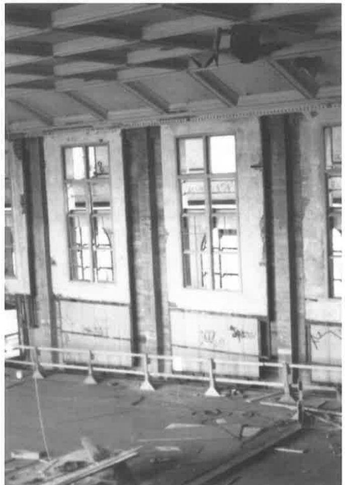
The south wall of Old Merritt's auditorium adjoins hallways in the classroom building on two levels. Transforming the auditorium to a senior center creates many design issues. The theater seats have been removed, the floor will be leveled, a kitchen area will be partitioned off inside, and door and window modifications follow. (Alfred Crofts)
