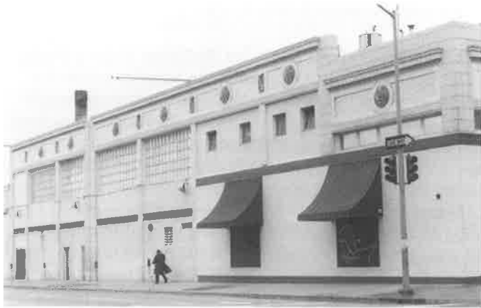
White tile-clad Swan's Market was built in several stages from 1917 on. This gradual assemblage is obvious on the 9th Street side, and creates some challenges for the reuse project. (Survey)
