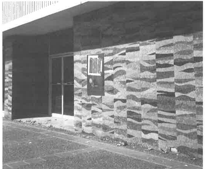
Preserving the recent past: Dahlke's remodeling of 1962-63 by architect Harry Bruno is a period design in its own right, and a reuse is being sought for these blue-green mosaics. (Betty Marvin)
