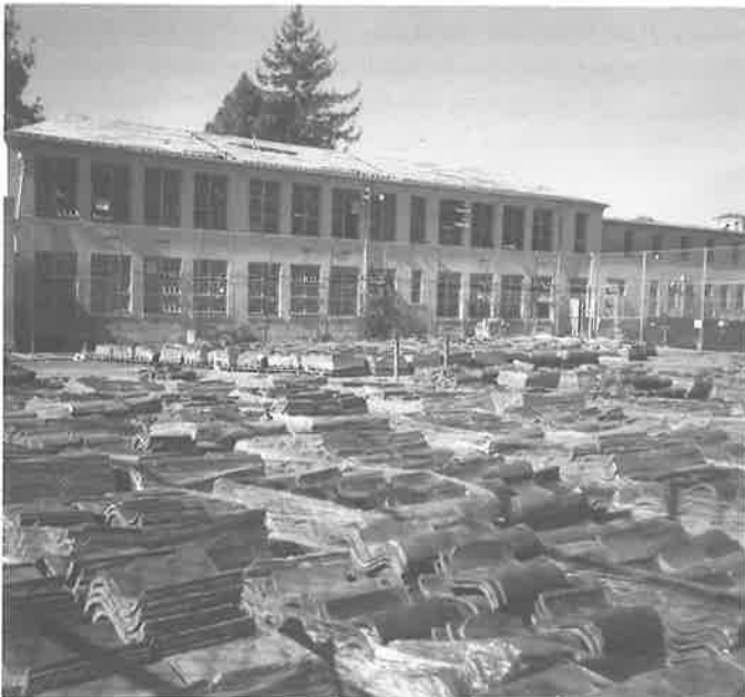
Recent rear view of Old Merritt showing roof tiles stacked and wrapped while roof is reinforced and repaired. (Betty Marvin)
