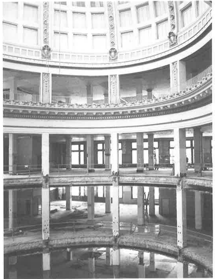
Ambitious rehabilitation job on the Rotunda was begun in the mid-1980s and has been interrupted by various financial and natural disasters. High tech reuse project now seems stalled. (Survey photo, c. 1985)
