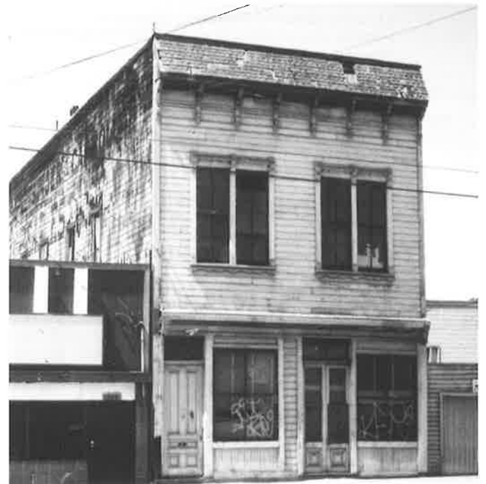
The Fruitvale Hotel was built about 1895, along the tracks opposite Fruitvale Station. This building type was important along 7th Street in West Oakland, but all examples there have vanished. Old wall signs read "Snetsinger & Carroll Real Estate" and "Fruitvale Hotel - Board - Rooms." Hotel has long been empty, and is now threatened with demolition. (Survey)
