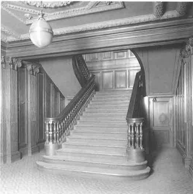
Have you seen this staircase? Parts from the Greene Library's magnificent entry have disappeared, to private hands or salvage dealers. Theft of features from unoccupied buildings is a serious problem; vigilant citizens can help. (Oakland History Room)
