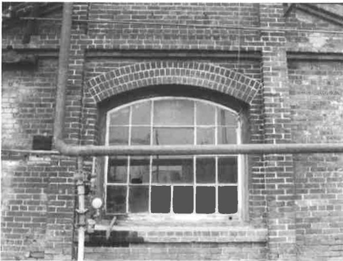
Southern Pacific Yards and Shops buildings, built between 1874 and 1914 and of supreme historical importance to Oakland and the west, will apparently be demolished since proposal to move them to Rio Vista Junction fell through for lack of time and funds. Caltrans told the railroad story in "Crossroads" video, and is also recording the buildings in HABS and other formats. (Fred Reichman)
