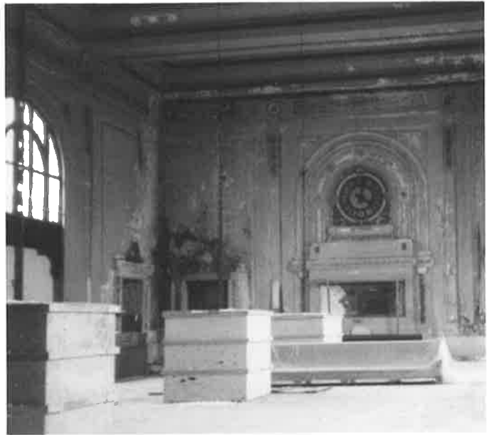
Southern Pacific station is approaching picturesque ruin status, if stabilization is not undertaken soon. You can help by writing to Metropolitan Transportation Commission in support of grant. (Betty Marvin)
