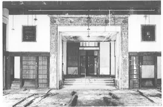
Years of leaking roofs nearly destroyed the library at Old Merritt, adding to costs for developers who now seek to restore the building. (Ken Rice/NOVA)
