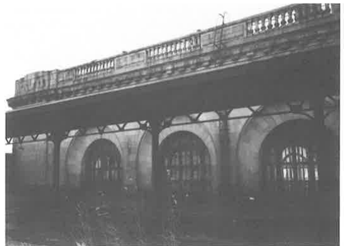
Inspectors climbed from the weed-grown Interurban platform behind the 16th Street Station and found the major source of damage to be clogged gutters. City is trying to bring about repairs. (Betty Marvin)
