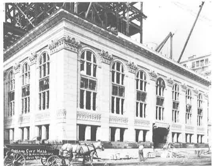
Construction photo of City Hall, dated July 3, 1912, shows steel frame of the tower, terra cotta cornice being attached, and other interesting details. Recent rehab was equally painstaking. (Oakland History Room)
