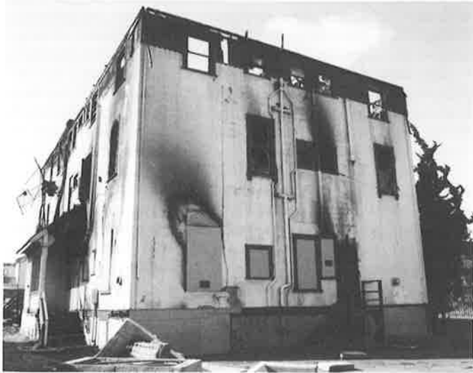
Wreckage of Miss Bisbee's School at 7th Avenue and Foothill exemplifies dangers to vacant buildings: can Preservation Element help? (Bruno Brandli)
