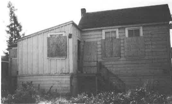
Landmarks Board and community groups are looking for a way to save the Mary Netherland house, predating the transcontinental railroad and associated with early black history. (Survey)
