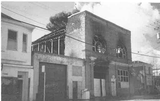
Oakland Point firehouse: while historic unreinforced masonry buildings are closed up awaiting retrofit, they are vulnerable to fire and other damage. (Oakland Cultural Heritage Survey)
