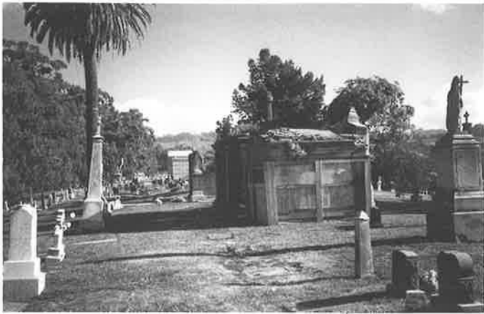
Peralta Mausoleum awaits resurrection in St. Mary's Cemetery. Rear view shows timbers shoring up the walls. (Betty Marvin)
