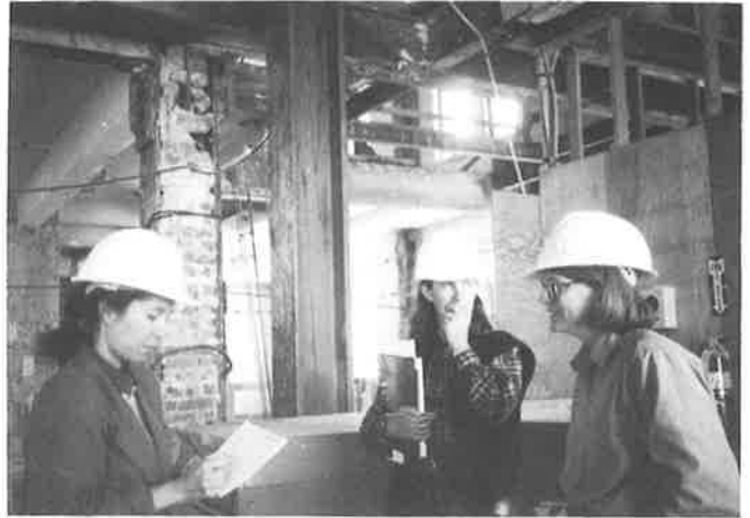
Helaine Prentice, Annalee Allen, and Veronica Martin tour the extensive seismic work at City Hall. Completion is expected in early 1995. (Betty Marvin)
