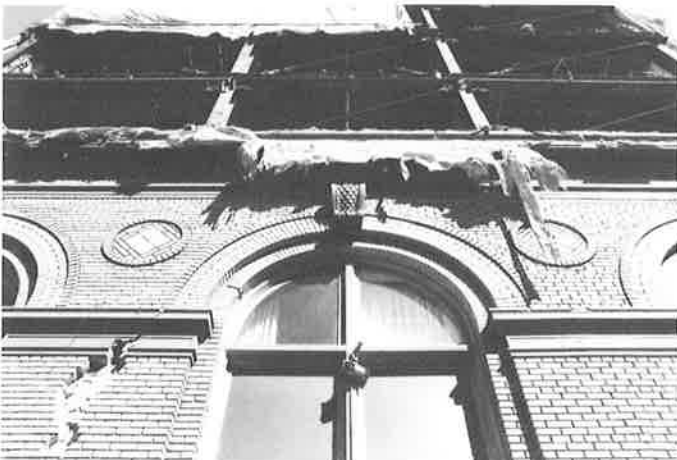
Earthquake damage in 1989 took four years to repair, but few residents were displaced. Work was recently completed by the Ratcliff Architects. (Phil Bellman)
