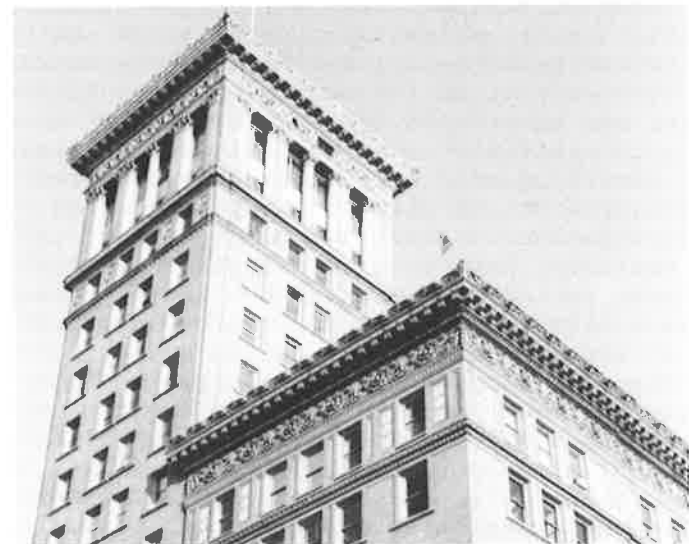
Elaborate terra cotta like the cornices of 1200 Broadway can be a maintenance problem; Board instructs owners that it should be cleaned and repaired, not painted. (Survey)
