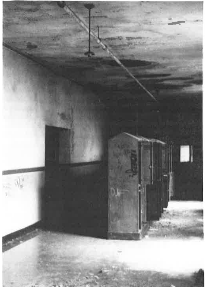
The hallowed halls of Old University High have been devastated by years of vandalism, water damage, and neglect. (Bob Brokl)
