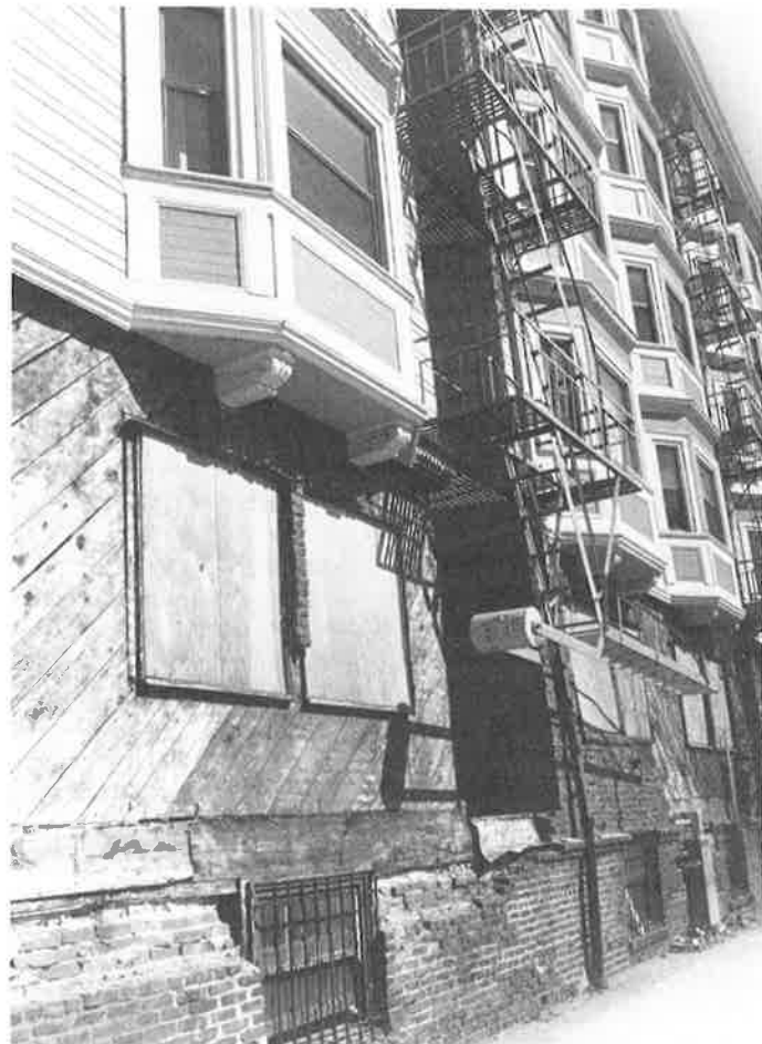
Earthquake damage to brick veneer at the Madison Park Apartments, 100 9th Street (C.M. MacGregor, 1908). EBALDC may return it to residential use. (Phil Bellman)
