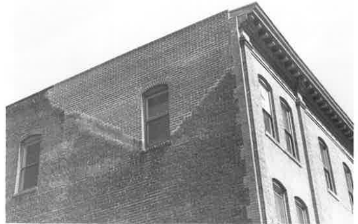
The Clay Building (former post office) at 10th and Clay: an encouraging example of a seriously damaged building which has been repaired. (Phil Bellman)
