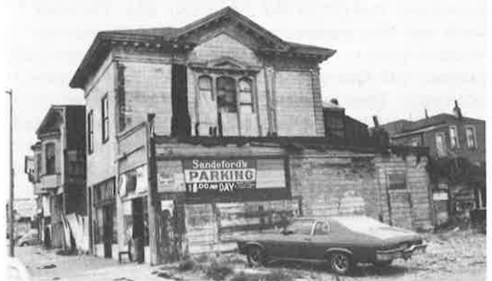
Surviving portion of Gibbons' Folly before the fire. The fire burned through the roof and damaged portions of the walls.
