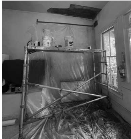
WATER DAMAGE on the ceiling got tackled in a recent effort to shore up infrastructure, above. At right is an ad from the 1930 Sacramento Bee .
