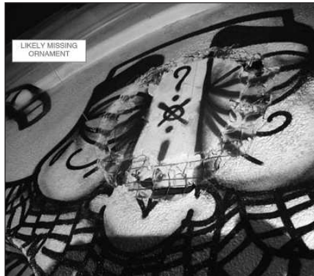
CLOSEUP of the graffiti face with a missing plaster ornament.
