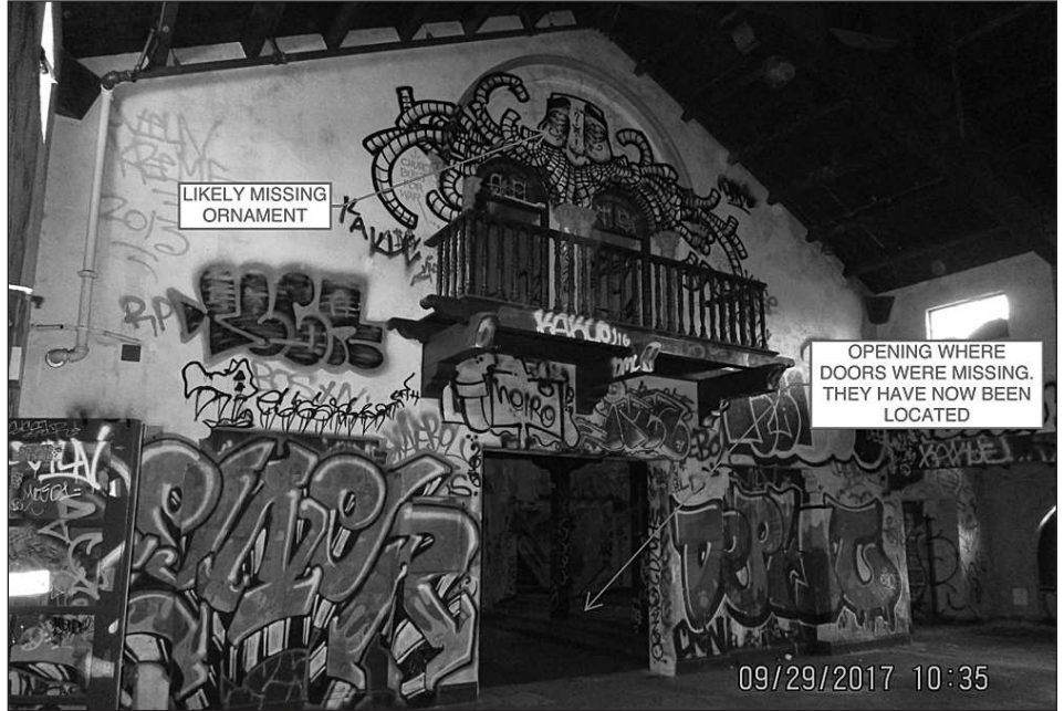
THE DINING HALL'S south side, covered in graffiti, shows intriguing vestiges of prior components, such as double doors and a missing ornament, as arrows show on the photograph.
