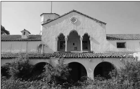
A MISSING RAILING once went through the columns end to end. There is an illegible reference to it on the plans, but we know it was there as there are holes and flashings. This is the east elevation.
