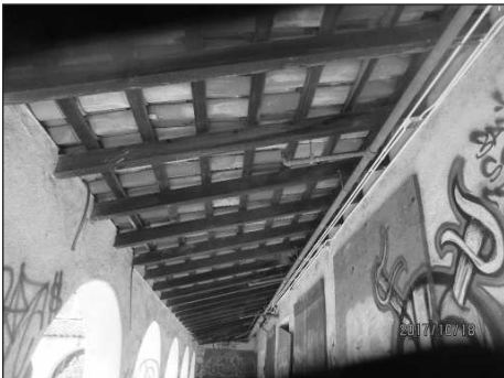
THE ARCADE ROOF. The plan is to salvage the batts and rafters for reinstallation.
