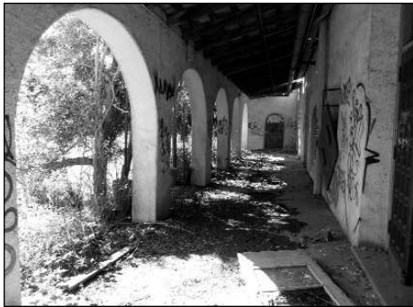
GRAFFITI AND DEBRIS mar a loggia off the planted courtyard.
